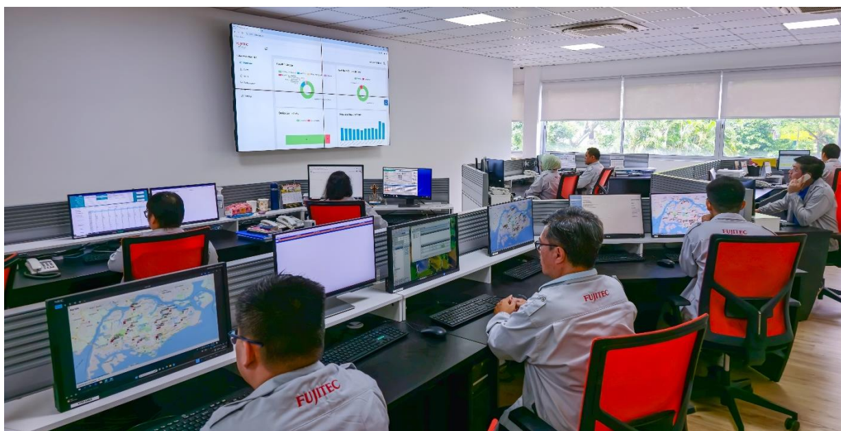
Remote monitoring system at Fujitec Singapore SafeNet Centre
