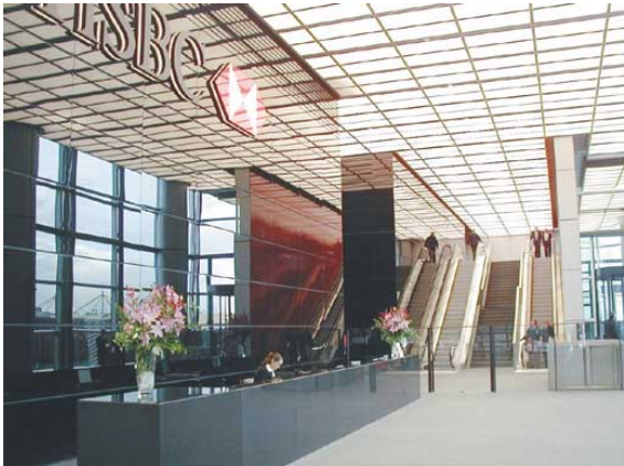
Fujitec escalators working at the headquarters building of HSBC in the United Kingdom
