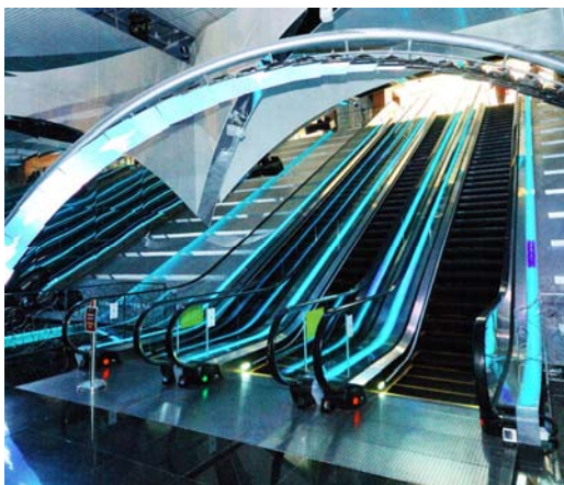
Escalators Serving “Resort World at Sentosa”
